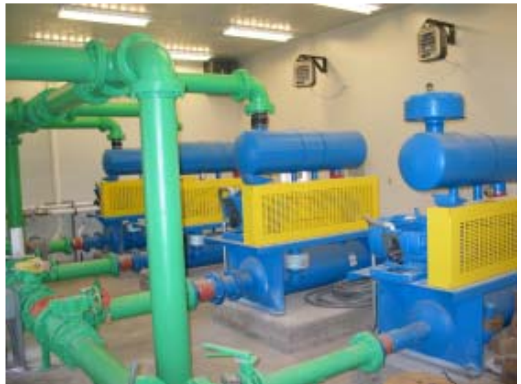
Wastewater facility at West Point, Nebraska.
