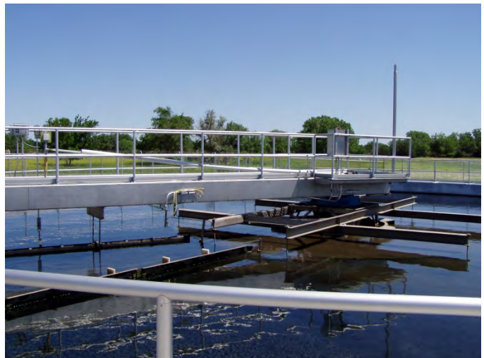
Part of Theresa Street Wastewater Treatment Facility, City of Lincoln.
