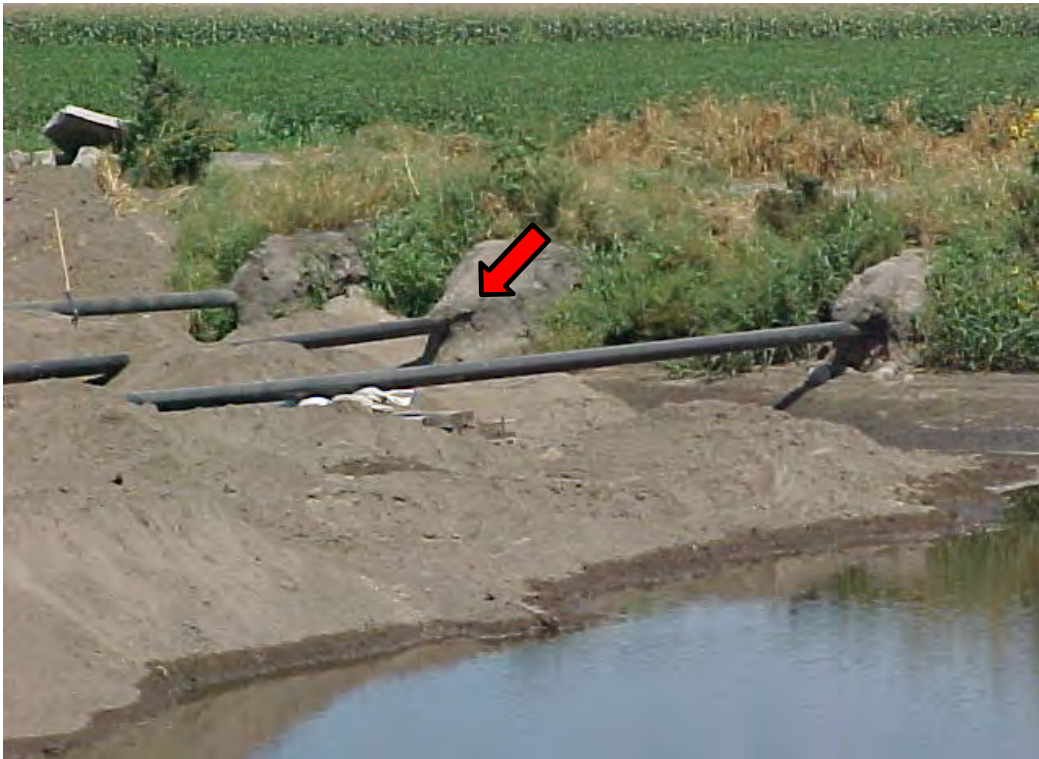
Excavation for ammonia pipeline repair and remediation. Arrow indicates adjacent ammonia pipeline, presenting difficulties for contaminated soil removal.
