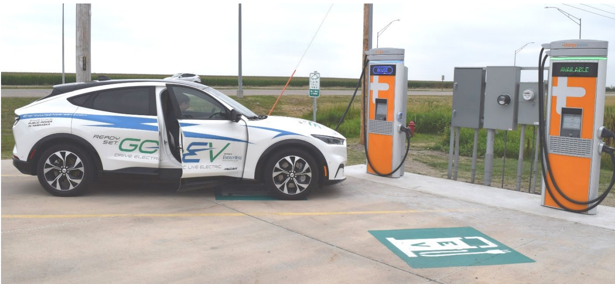
Two DC fast electric vehicle chargers at the York, Nebraska station installed by the Nebraska Public Power District.
