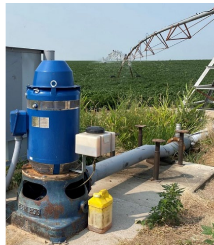
New electric motor at wellsite.
