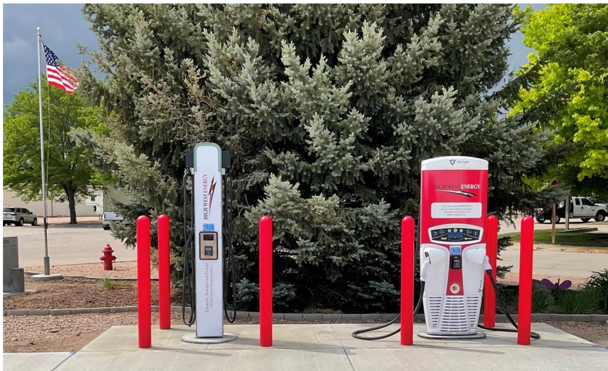
Level 2 (left) and DC fast charger installed at the High West Energy Service Center in Potter (2 miles from Interstate 80 in western Nebraska) and partially funded through the Nebraska Electric Vehicle Charging Rebate Program. Photo courtesy of High West Energy.
